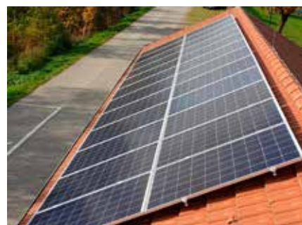
Photovoltaik FZA St. Andrä
